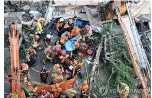
Building collapse accident
